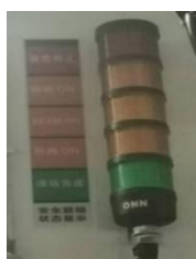
Fig.4b Sound and light alarm lights
